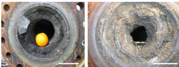
Figure 2. Photographs of scales in surface pipelines downstream of the orifice plate. The scale bar is 10 cm.
